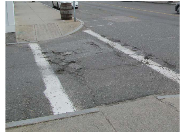
Crosswalk pavement is deteriorated.
