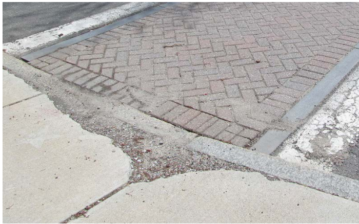
Crosswalk ramps are deteriorated.
