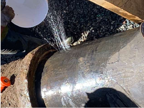
Water main leak
